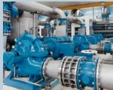
Pump, Fans, Compressors
